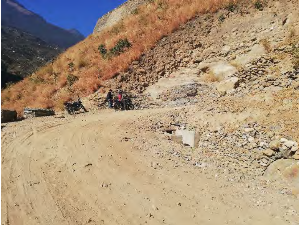
Photo 11: Chainage 1+100. Hairpin bend could require further slope stabilisation
