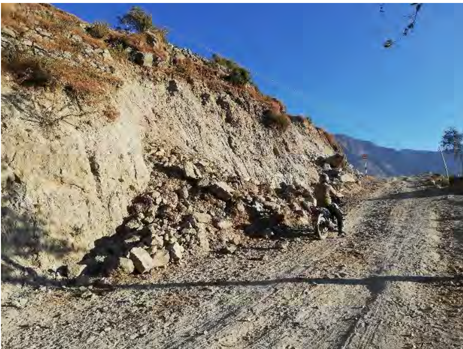
Photo 10: Chainage 12+460. Observed landslide.
