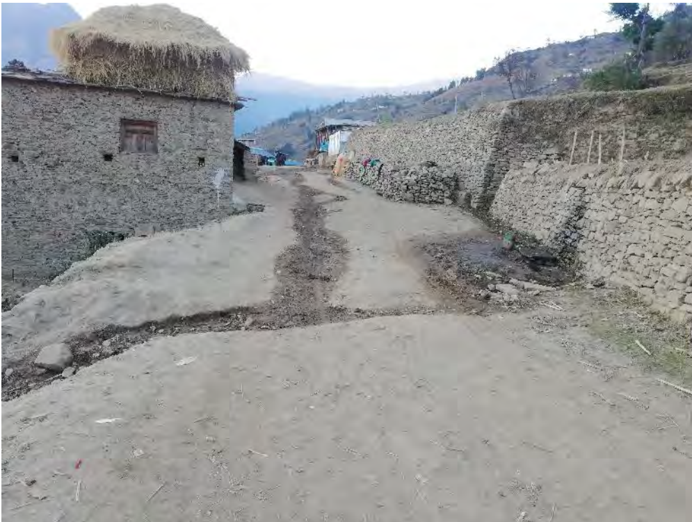
Photo 13: Chainage 15+900. Minimal side-drain and stone piling. Pipe required for water drainage.
