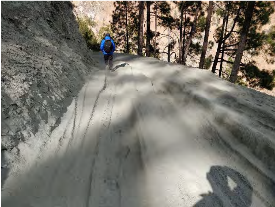
Photo 21. Chainage 10+650. Dusty sections of road.
